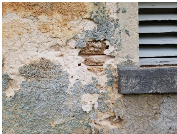
Figure 66 View of calcarenite showing inappropriate surface render
