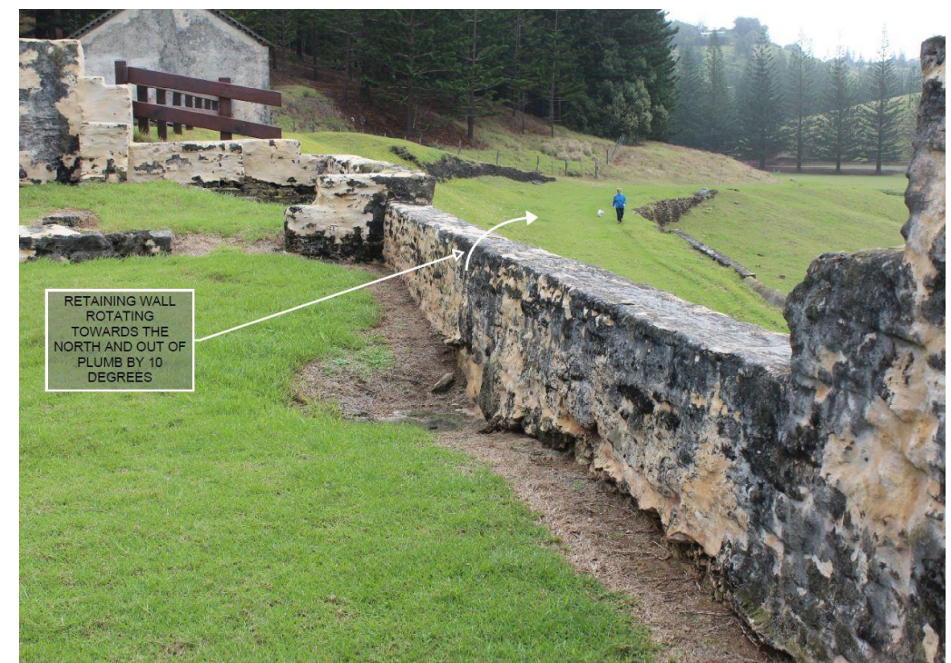
Northwest retaining wall showing rotation.
