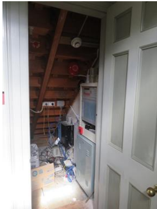
The stair in the Old Military Barracks is timber and not fire rated. The switchboard under the stair is a potential fire source.
