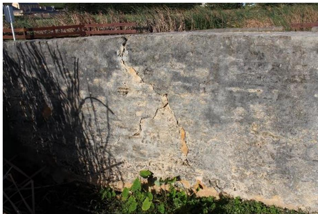
Crack pattern on the western side of the Bounty Street Bridge.
