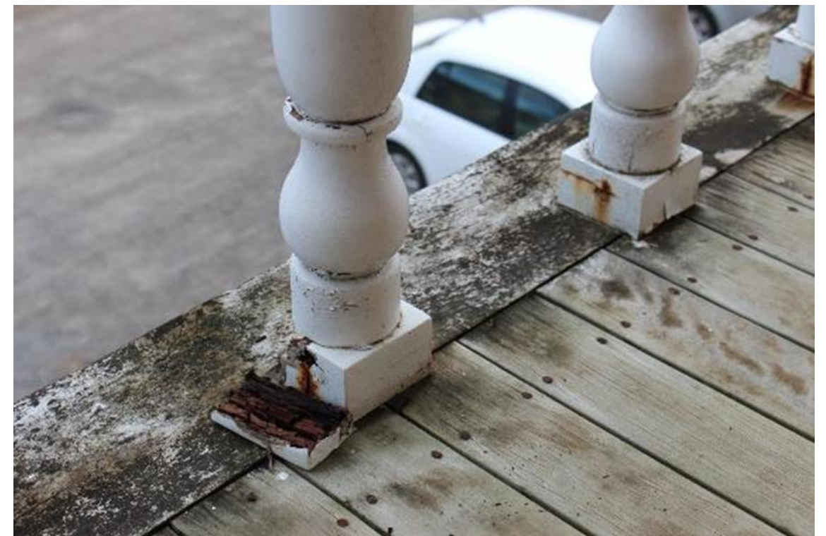
Decayed timber on vertical members of balustrade.
