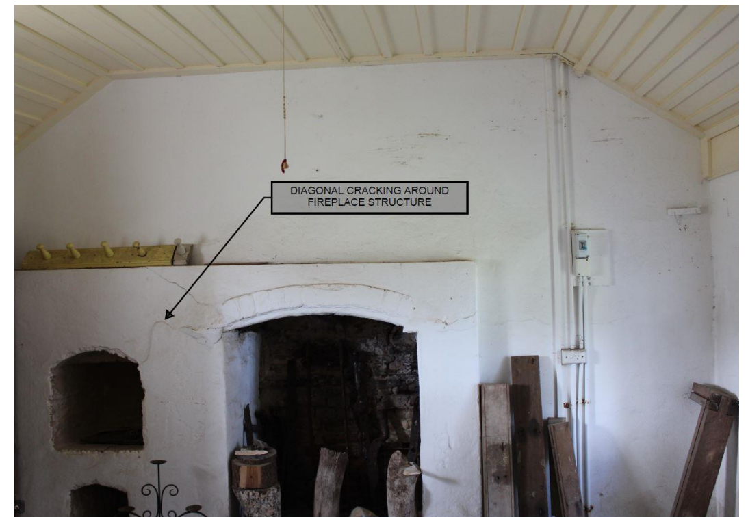
Internal wall cracking in Surgeons Quarters Kitchen.
