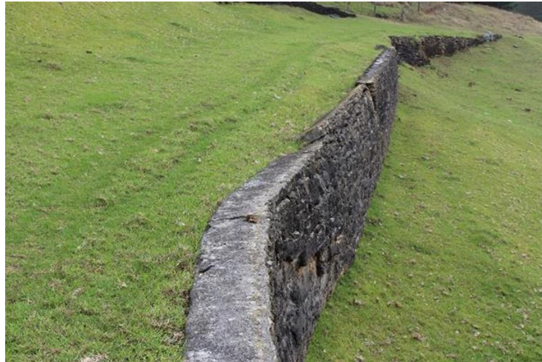
Bulging retaining wall below Civil Hospital.
