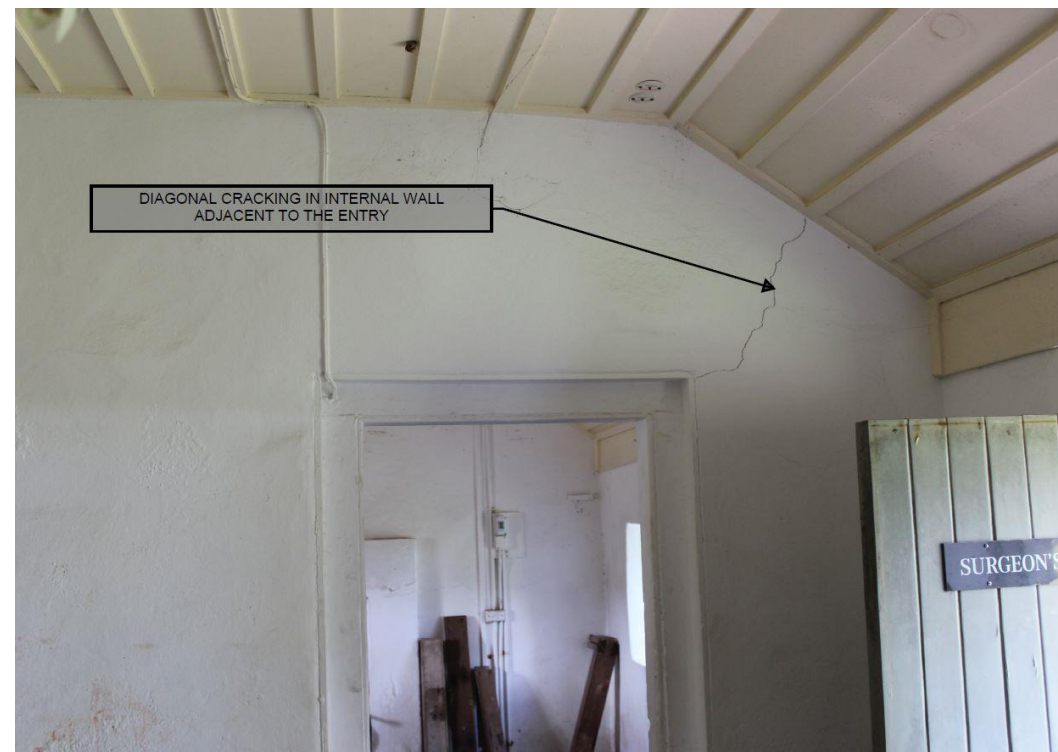
Internal wall cracking in Surgeons Quarters Kitchen.
