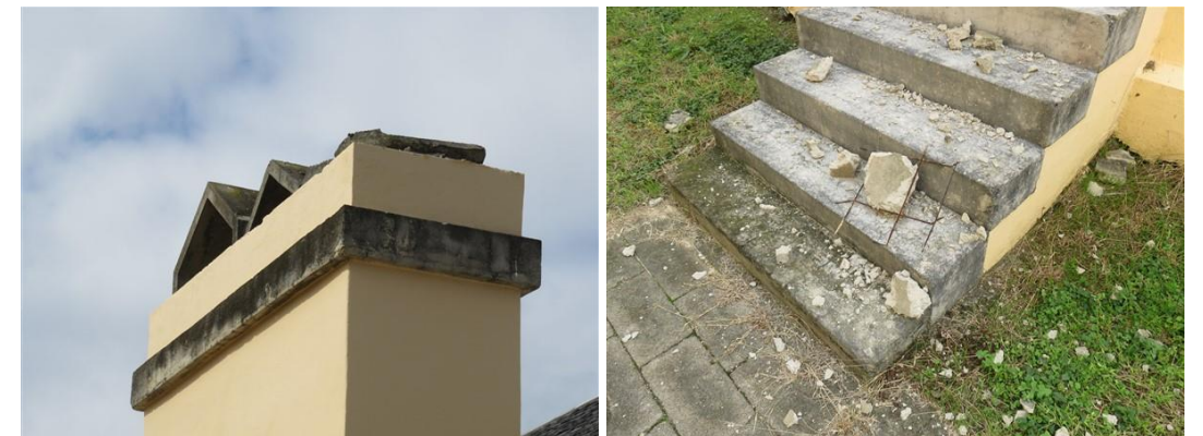
Failed reinforced concrete chimney caps which have fallen on the entrance steps to the neighbouring building, Old Military Barracks, 4 May 2018.
