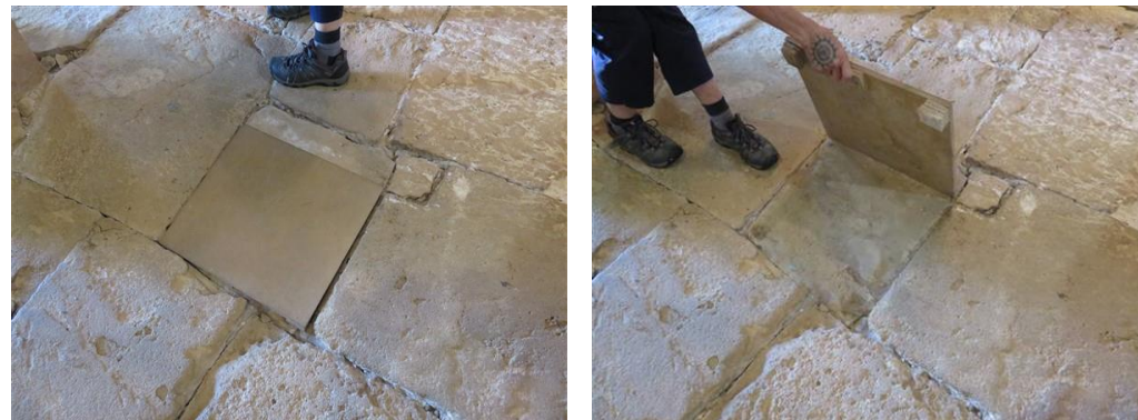
Plywood infill panel to level a hollow stone in the floor of the Commissariat Museum.
