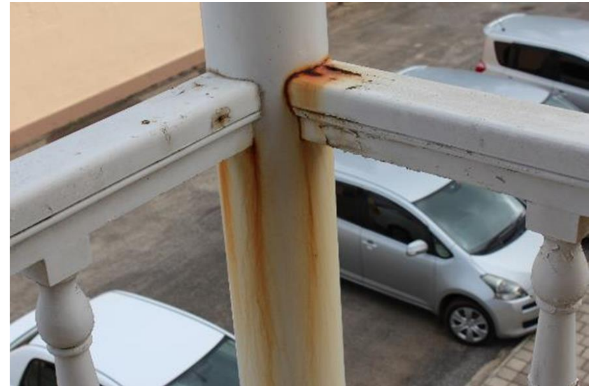
Corrosion staining on timber post from rusting steel fixings.
