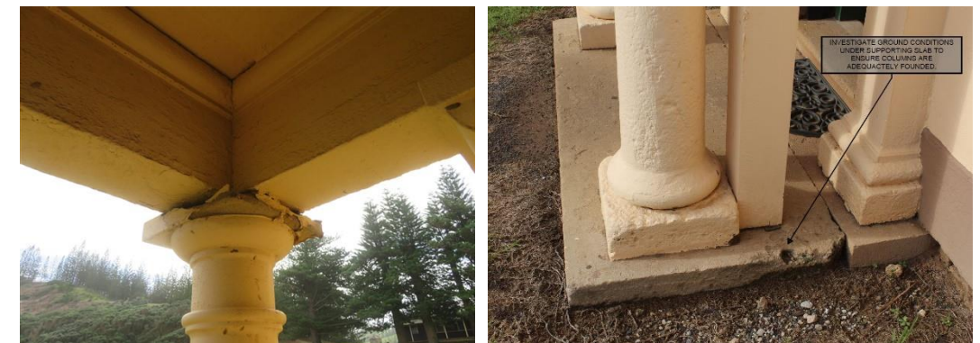
Decayed northern column capital and stone base to REO portico.
