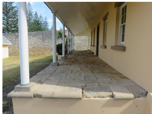
Decayed margin stones may need replacement to provide protection to the verandah walls, Old Military Barracks.
