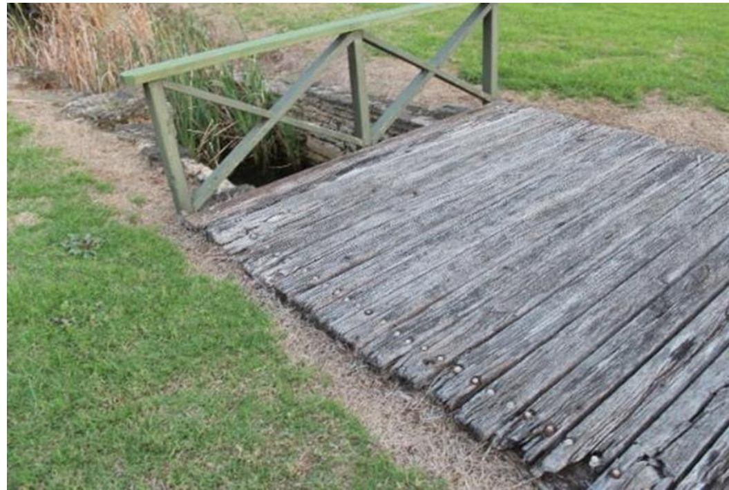
Decayed timber members spanning across the creek channel in the Government House Reserve.
