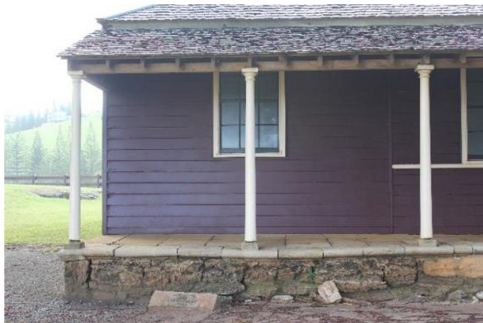
Southwestern end of verandah showing subsidence.
